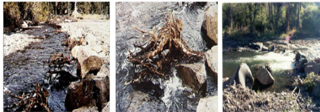
To improve pool quality and quantity, the Columbia Soil and Water Conservation District has installed rootwad revetment (left), large organic debris placement (middle), and vortex weirs (right), in the Tucannon River. (Photographs: Courtesy of the Columbia Conservation Soil and Water Conservation District)
