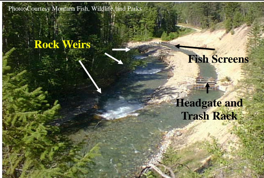
To improve fish habitat, and associated populations, weirs, screens and headgates were installed in Graves Creek.
