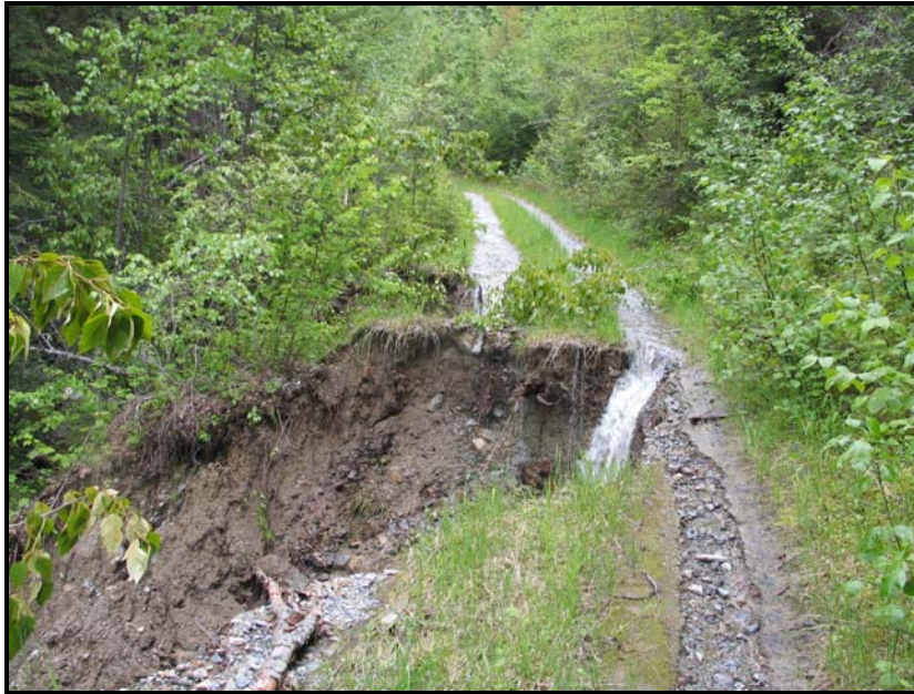
Skidoo Creek flowing down a logging road before eroding the road prism and returning to the main channel.
