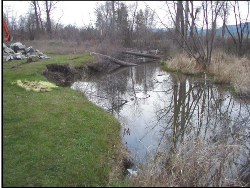
Eroding vertical bank on Dayton Creek prior to reshaping.
