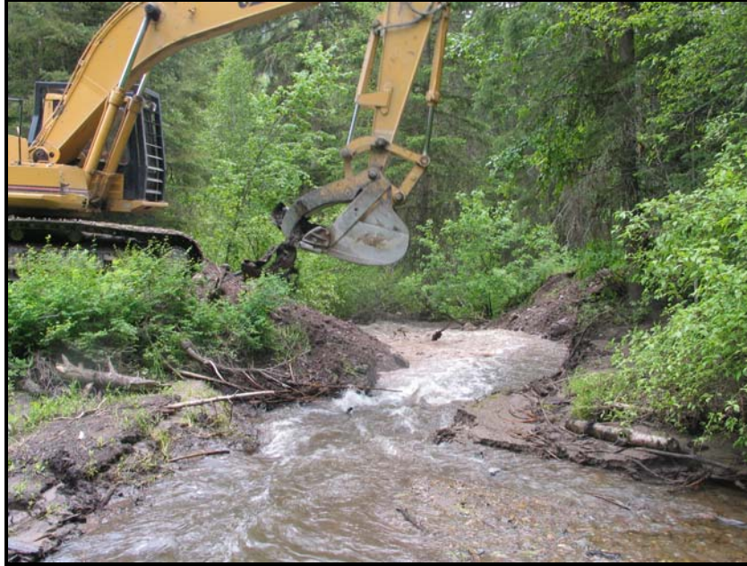
Removal of perched culvert on a tributary to North Fork Jocko River, 2005.
