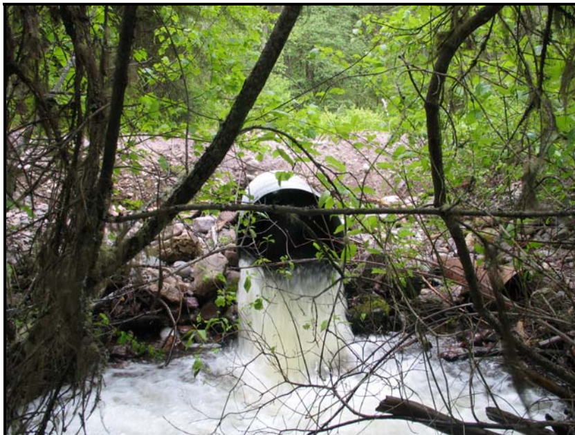
Perched and undersized culvert in tributary to North Fork Jocko River, 2005.
